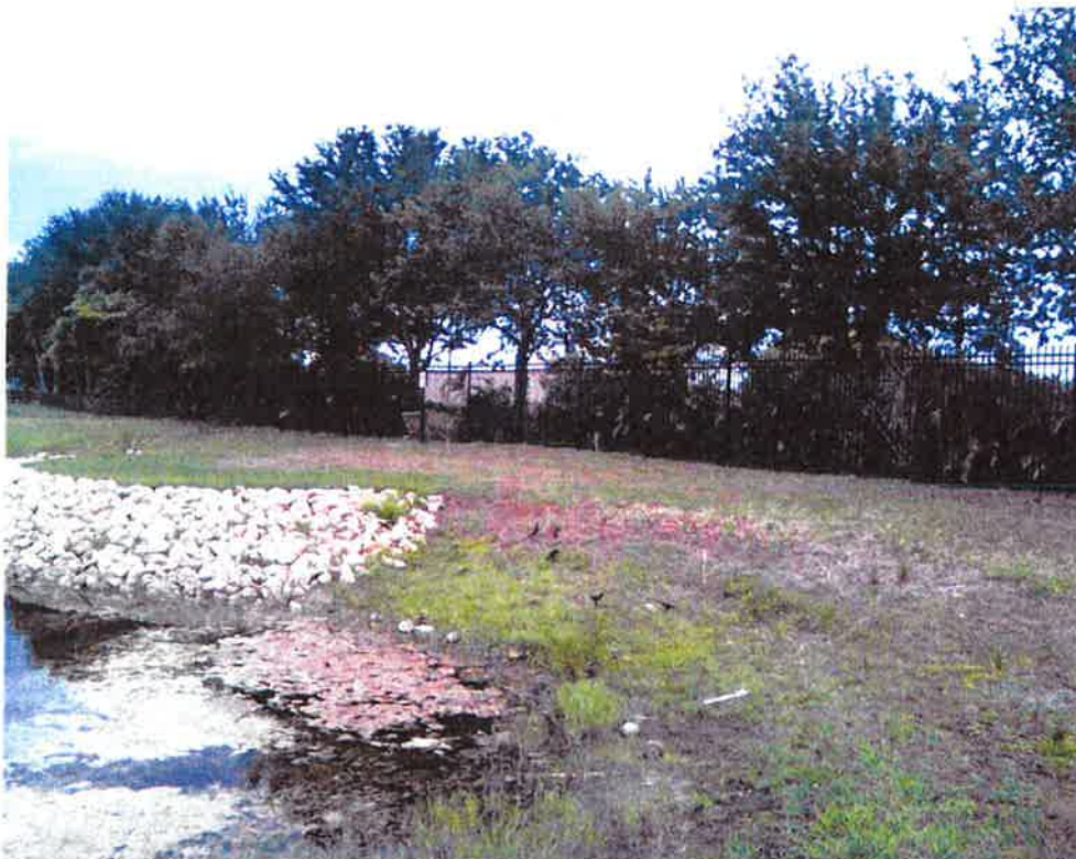
Figure 28 – East End of Lake 7 at Outfall Structure Looking at New Fence on 05/29/2015
